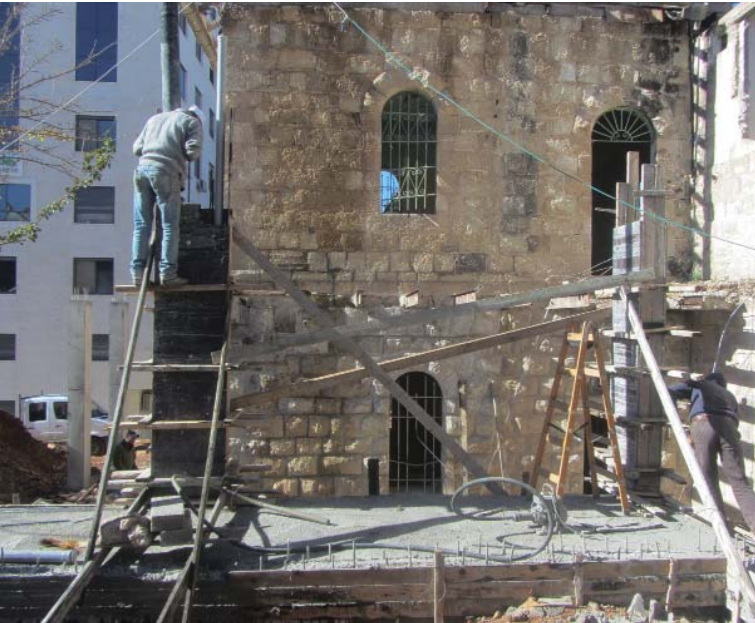
Construction of a nursery school in a Greek Catholic school in Ramallah, Palestine.
