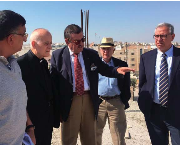
The Delegation of the Grand Magisterium and representatives of the Patriarchate at the construction site of a church in Jubeiha on the outskirts of the Jordanian capital, with the architect in charge of the work.
